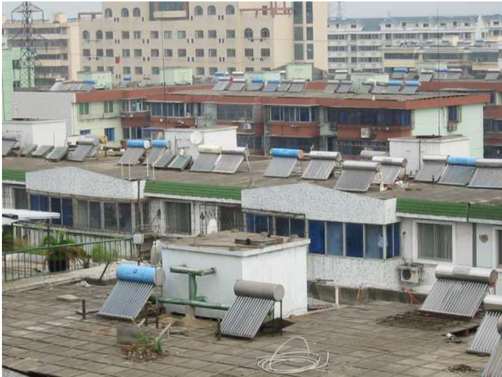
Figure 22: Example installation showing lack of building integration of solar heating in China
